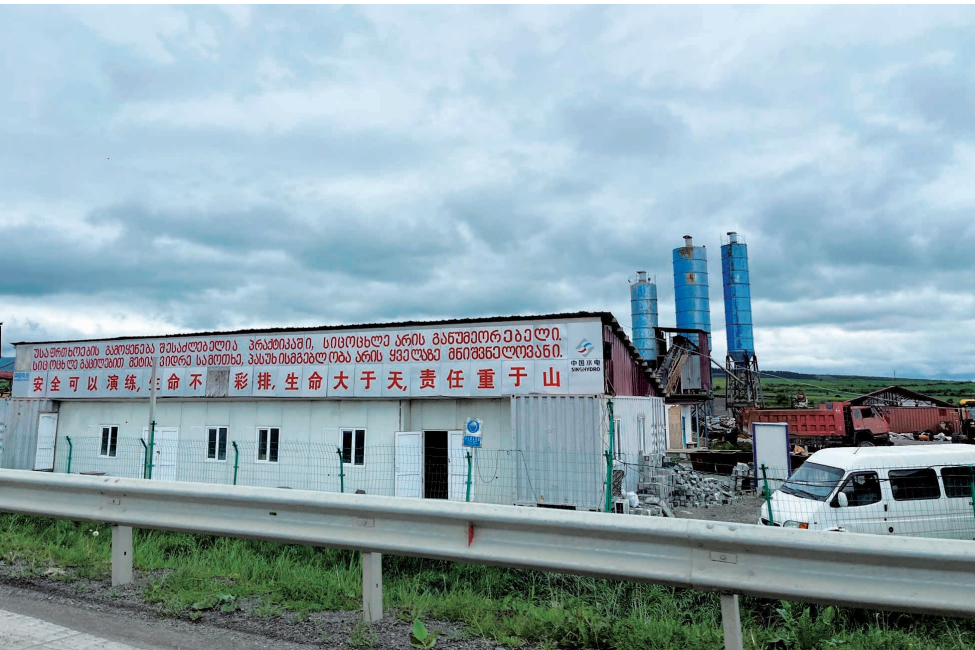
Base camp of a Chinese construction company in the Rikoti road construction project in Georgia.
